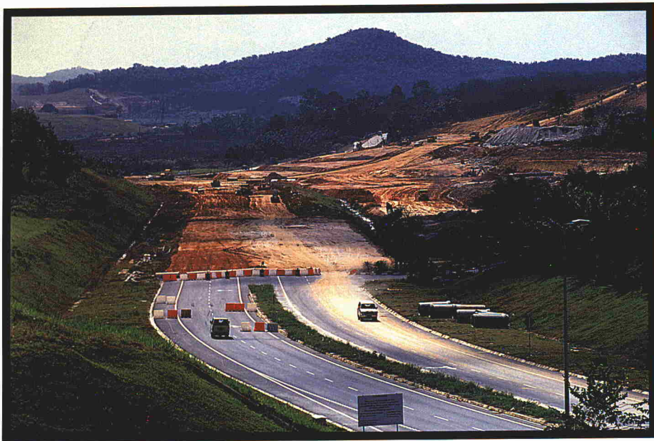
INFRASTRUCTURE WORKS IN CYBERJAYA, INFO-TECH CITY IN THE HEART OF THE MULTIMEDIA SUPER CORRIDOR, NEXT TO PUTRAJAYA FEDERAL GOVERNMENT ADMINISTRATIVE CENTRE
